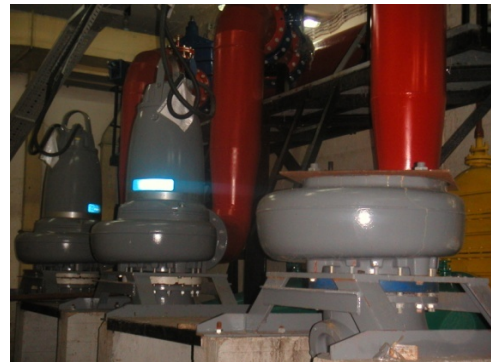
Photo2-2. Pump facility for waste water discharge
