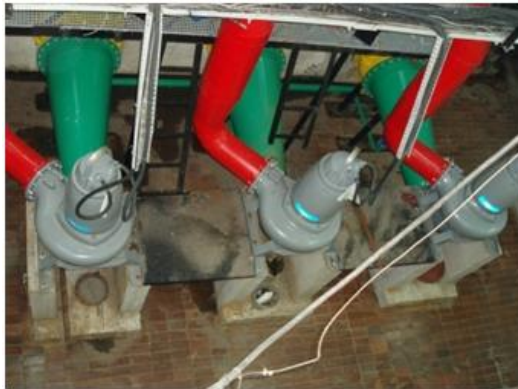
Photo 2-1. Pump facility for storm discharge
